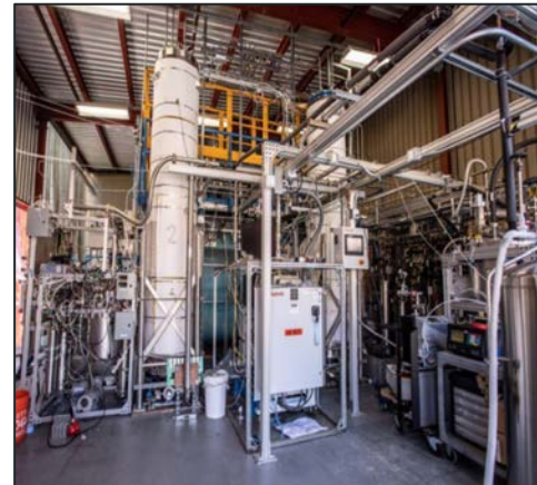
Kr-removal system at SLAC, CA
